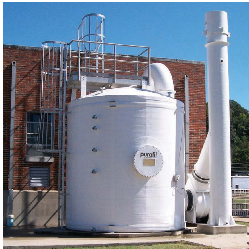
Moccasin Bend Wastewater Treatment Plant, Chattanooga, Tennessee
