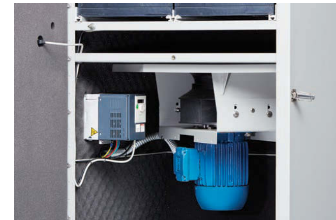
Blower access with safety switch
